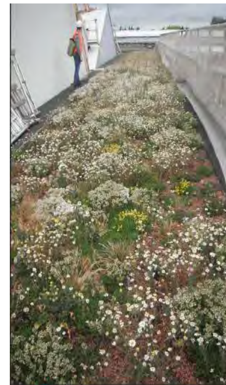
Fig 7 Green roof, Ruislip, susdrain.org
